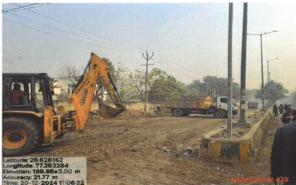
Figure 1: Site Photograph of Mixed Waste on Roads.
